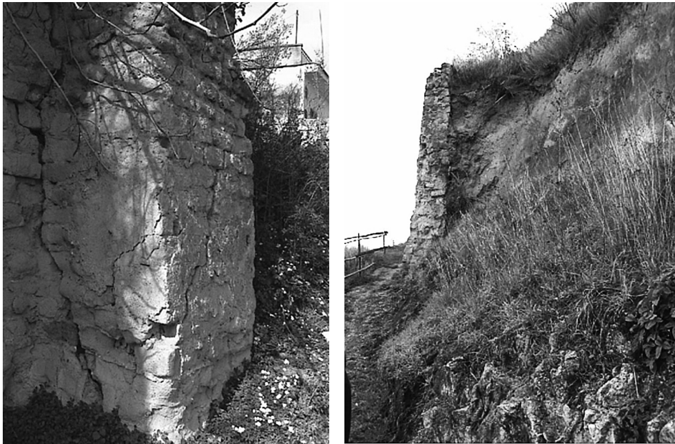
Fig. 9. Examples of deterioration of the system of retaining structures; left: detachment and fracturing of a counterfort; right: collapse of a retaining wall
