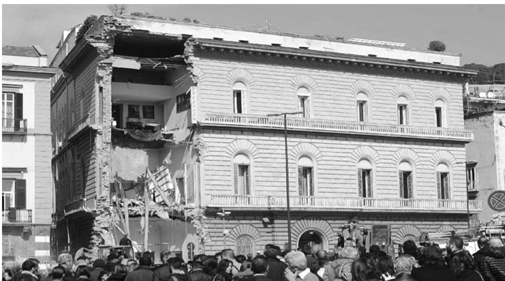
Fig. 30. The collapse of the western corner of the Guevara di Bovino Palace, Napoli
