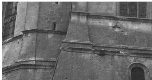
Figure 16. The cornice displacement shows the apse settlement.
